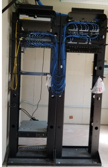
Networking equipment. Always on!
