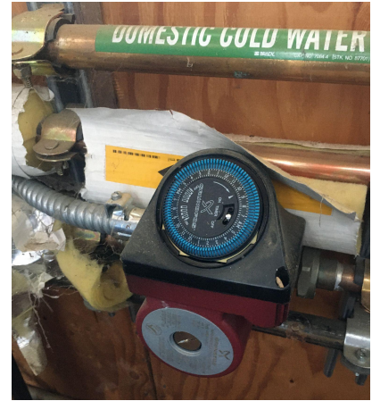
Water heater pump
