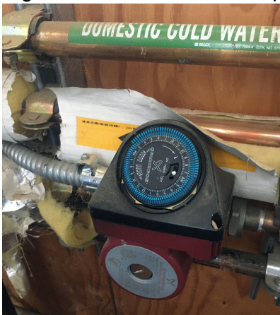
Figure 11: Water Heater Pump
