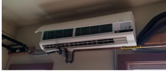
Figure 3: Server Room Wall-Mounted AC Unit
