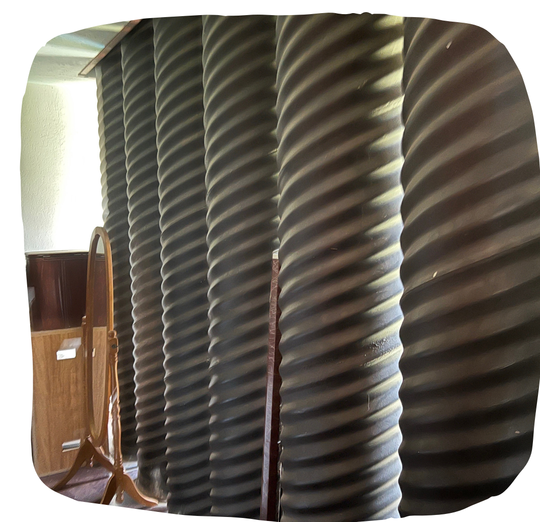
Thermal storage tubes
