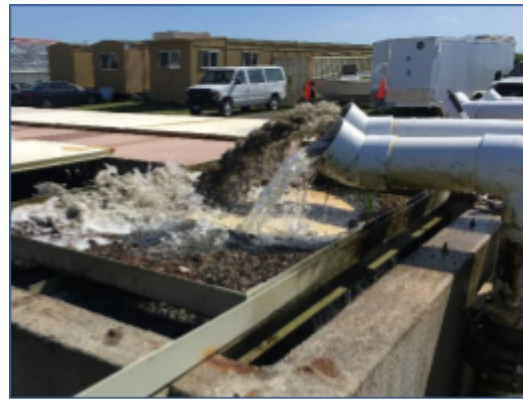
Figure : Primary separator for influent pouring into the clarifiers
