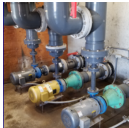
Figure : Three pumps sending seawater to rooftop holding tanks at BML facility
