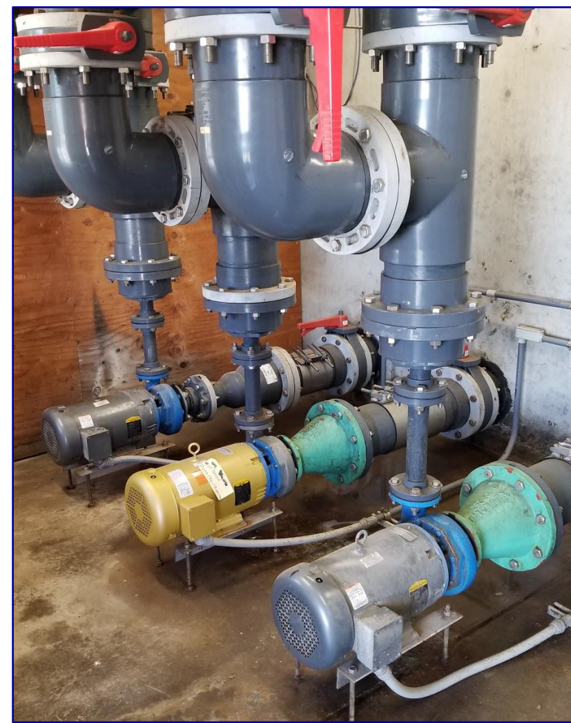
Figure 1: Pumps to holding tanks representing sizeable energy use
