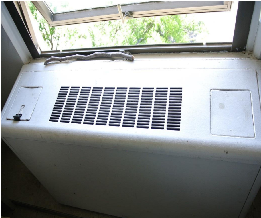
Figure 3.1-1 Existing Fan Coil Unit
